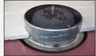
Fire Rated Ceiling Valve sealed after a fire.
