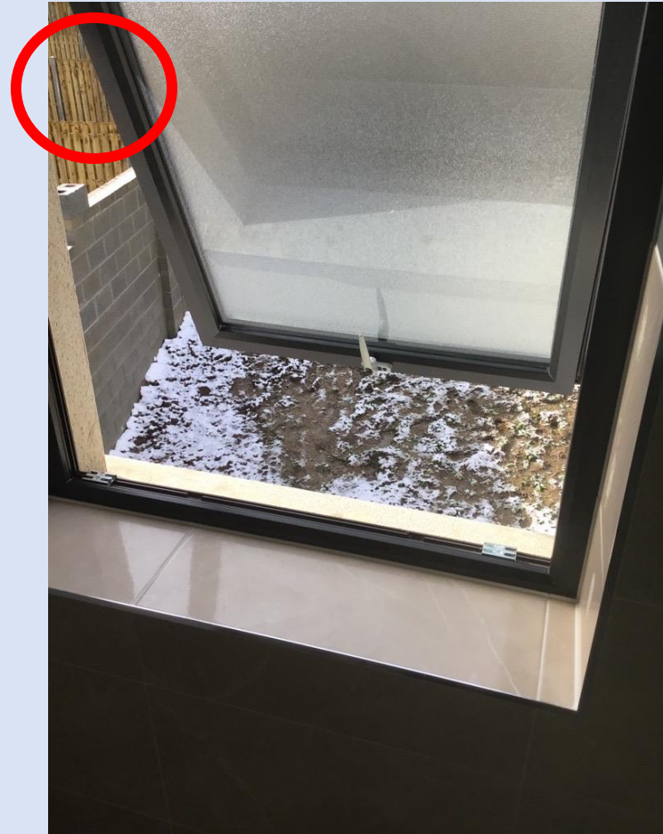
Safety restrictors required
