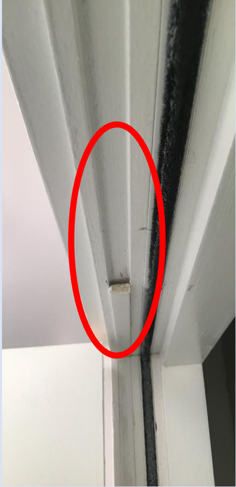
Intumescent strip has fallen out
