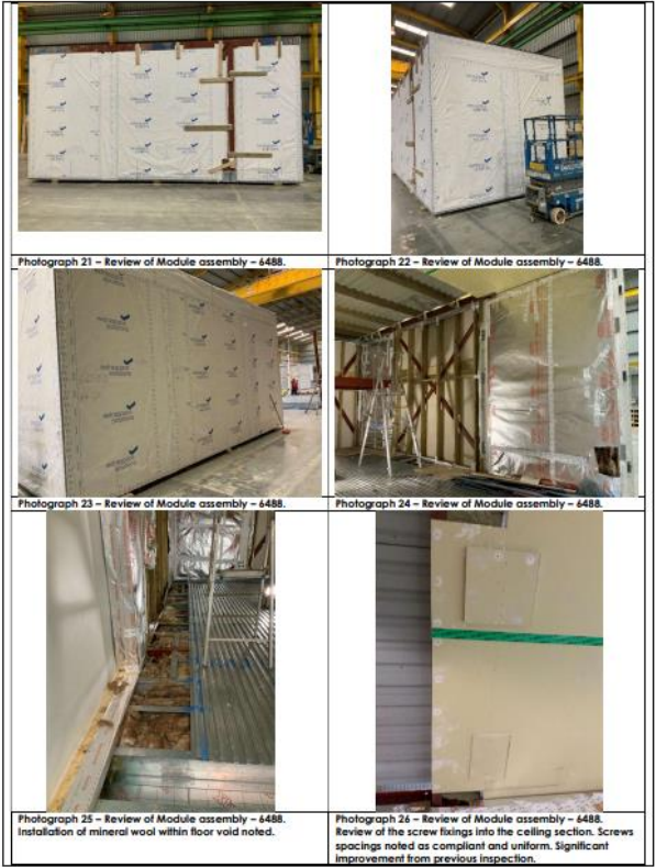
Factory Inspection of a Modular construction used in a recent Healthcare Project
